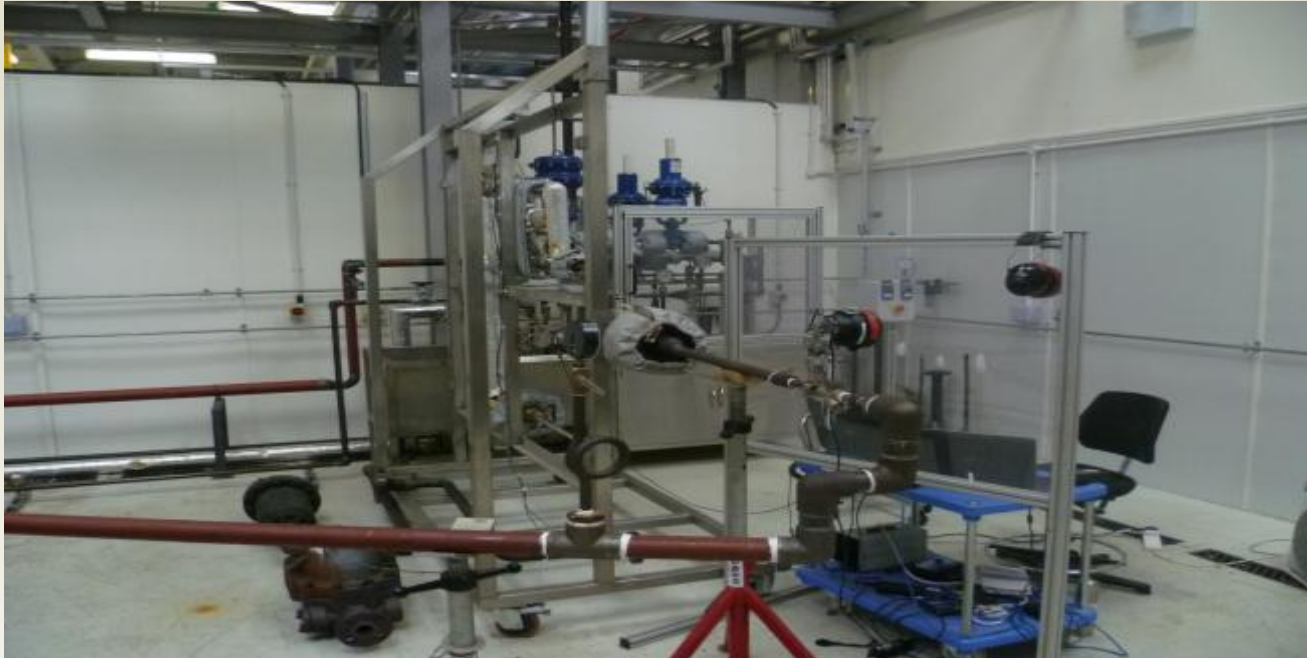
20 - 60 Bar Steam Meter test set up
