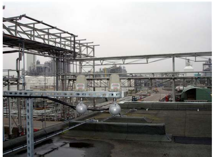
Hexion uses Honeywell wireless transmitters for wireless smoke detection and control room communication.
